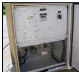
Power Transfer Module
